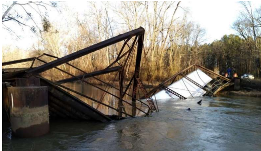
(a) The Dale bend bridge in USA, a truss bridge built in 1930
